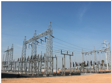
High Voltage Substation
