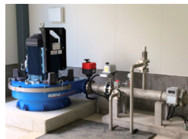
Small Hydric Generator
