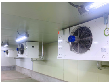
Freeze Room System
