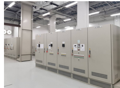
Low Voltage Substation
