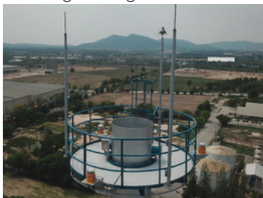
Lightning Protection System
