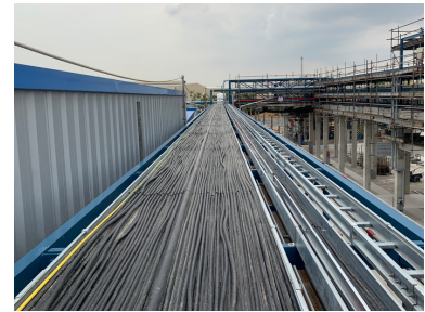
Wiring Power system
