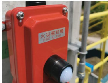
Fire Alarm System
