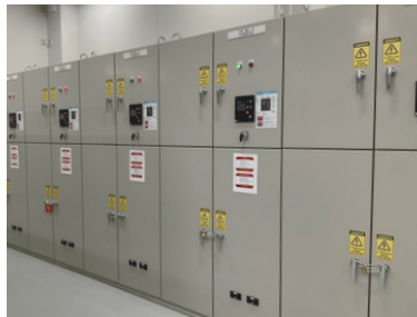
Medium Voltage Substation
